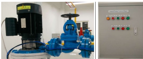
Figure 3: Liquid cargo pump system
